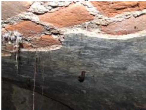
45. Loose and missing plaster to soffit of vaults
