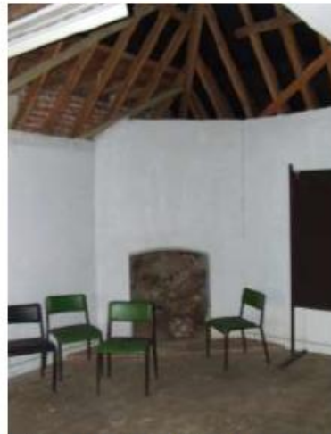
24. General view of first floor room. Flue above fireplace has been removed.
