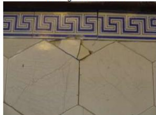
14. Cracks to tiles
