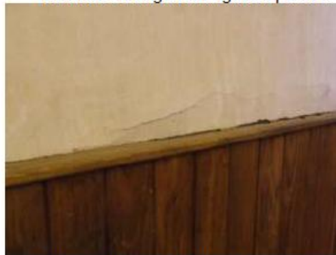
20. Cracking to plaster above timber cladding
