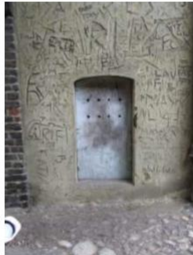
6. Vandalised rendered infill panel
