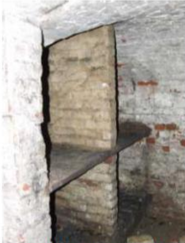
43. Slate storage shelves
