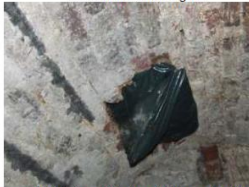
46. Hole in soffit of vault 'plugged' with plastic bag.
