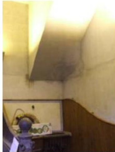
16. Staining to ceiling and wall plaster
