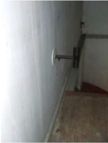
29. Handle to operate ventilation shaft
