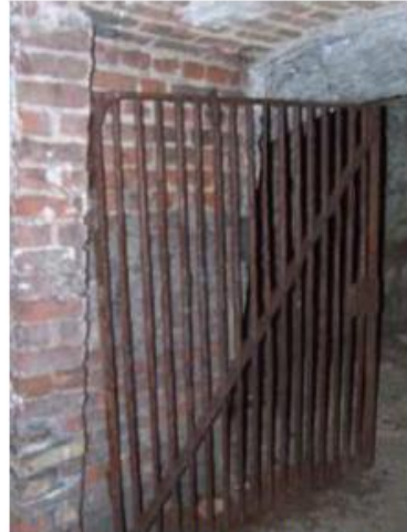
44. Corroded metal gate
