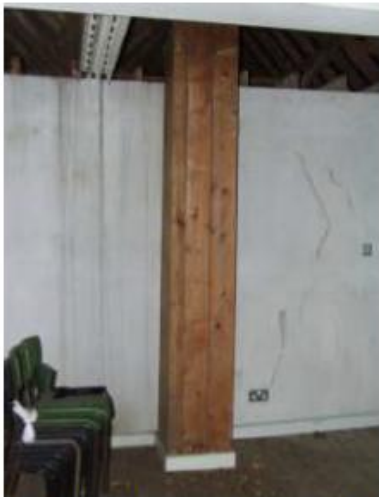
27. Timber clad ventilation shaft to first floor room. Terminates above ceiling finish.
